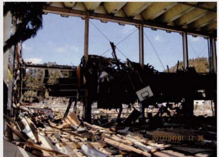
Only the frame of the gymnasium survived
