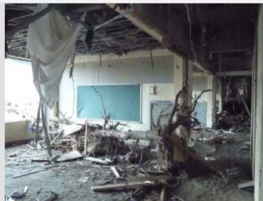
Wall is lost due to water pressure
