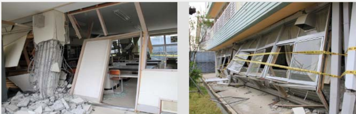
Collapsed pillars and walls (school facilities built according to the old quake-resistance standards)
