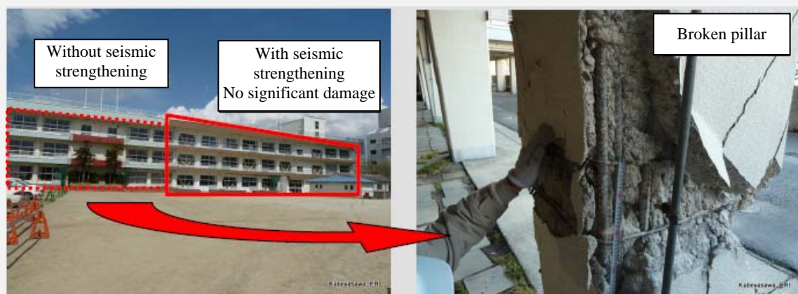
Comparison of the damage to the part with seismic reinforcement with the damage to the part without reinforcement (Seismic retrofitting for the damaged part had been scheduled for the next year.)
